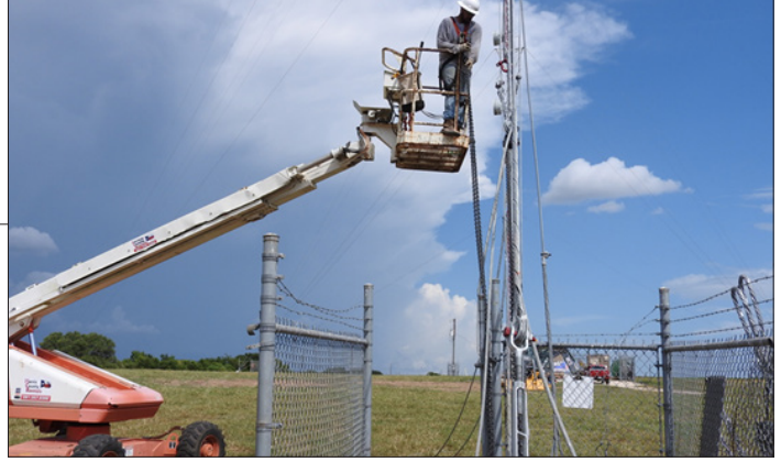
What not to do? Incorrect fall protection, standing on rails.
