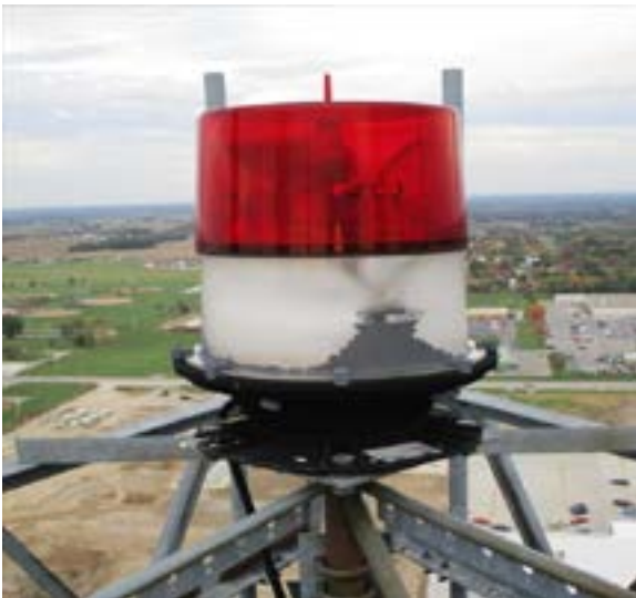
(Crazing of flash head, affecting FAA intensity requirements, needing a replacement)
