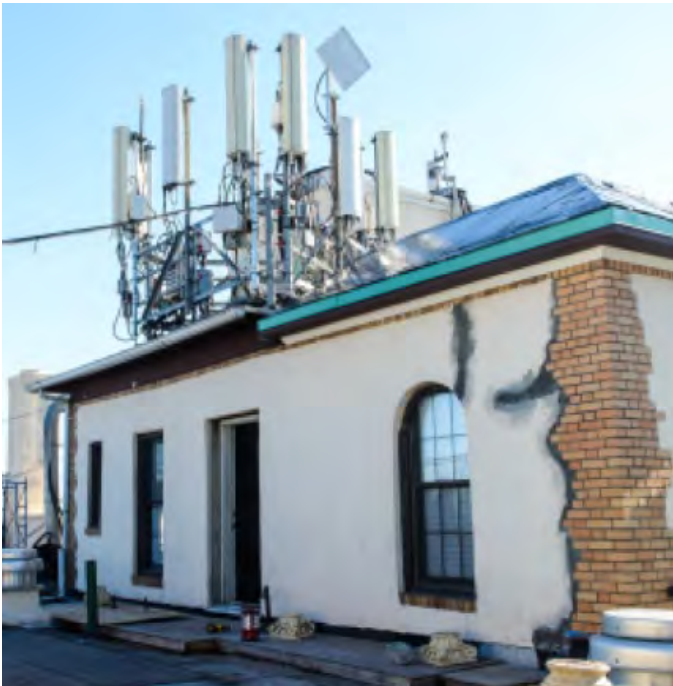
Figure A.b.4: Custom penetrating rooftop mount installed on penthouse roof
