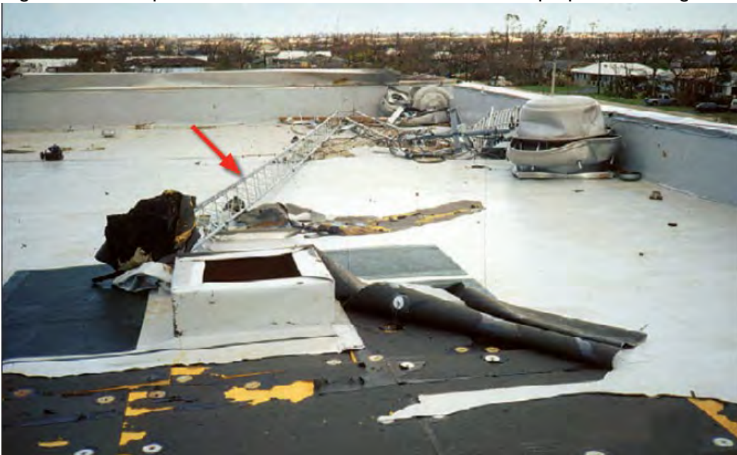
Figure B.5: Collapse of roof mounted antenna tower including progressive peeling of the roof membrane (Reference: FEMA 543 Risk Management Series: Design Guide for Improving Critical Facility Safety from Flooding and High Winds (January 2007))
