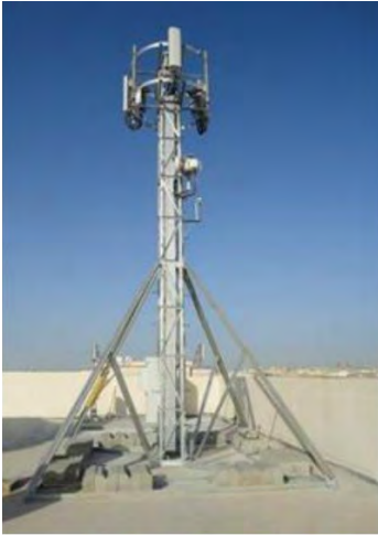
Figure A.d.1: Small Lattice Tower ballasted on corner of a building roof
