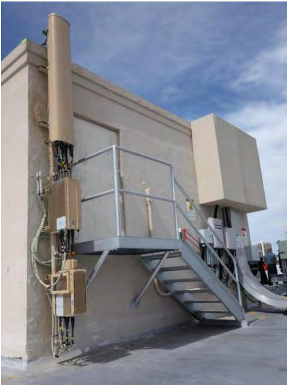
Figure A.a.2: Wall mount installed on the penthouse wall of a building
