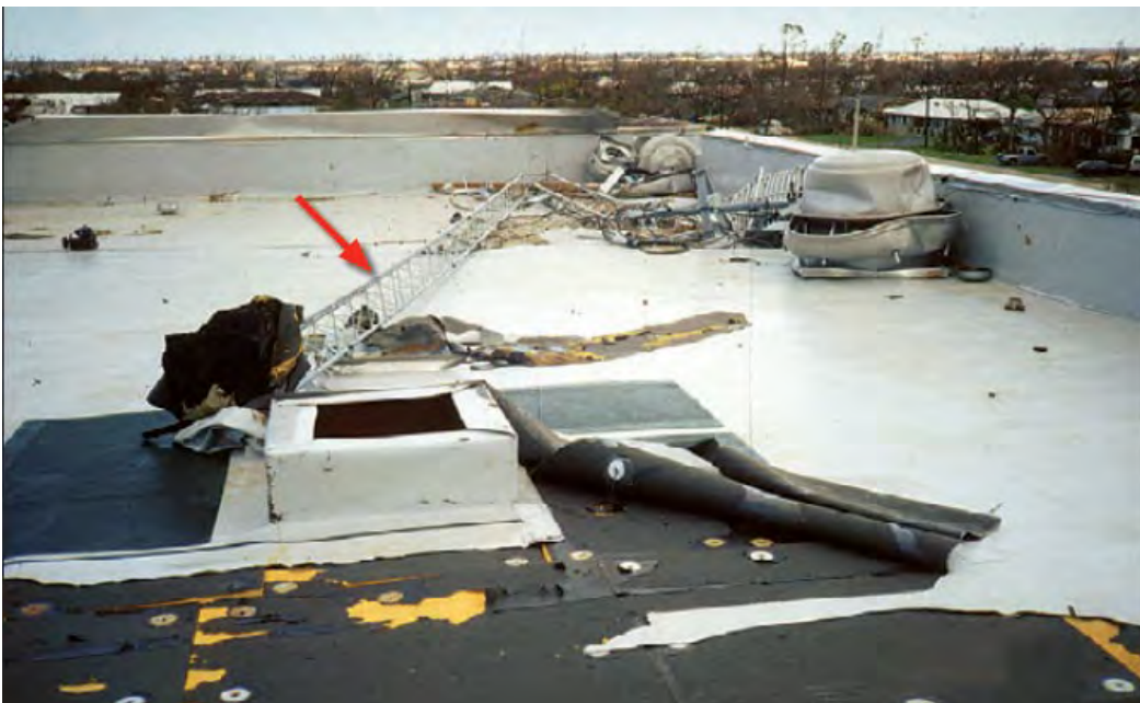
Figure B.5: Collapse of roof mounted antenna tower including progressive peeling of the roof membrane (Ref: FEMA 543 )
