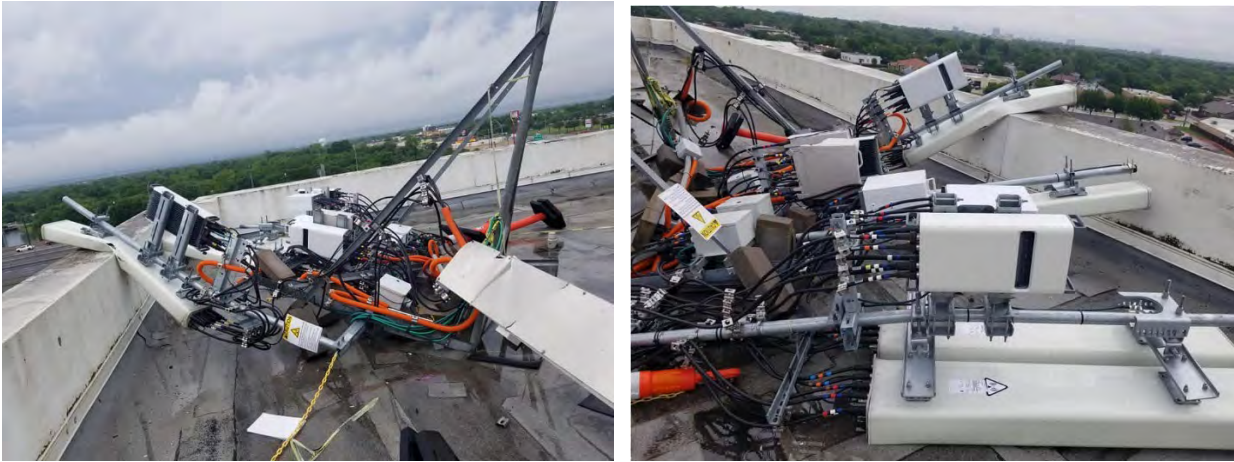
Figure B.1: Rooftop sled-mount frame overturned as a result of not having enough CMU blocks
