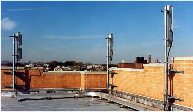
Figure A.a.4: Pipe wall mount installed on parapet wall of a building
