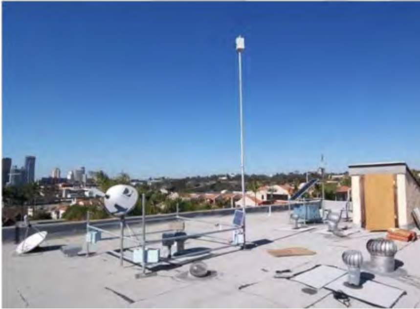
Figure A.b.1: Custom penetrating mount supporting radio and dish equipment
