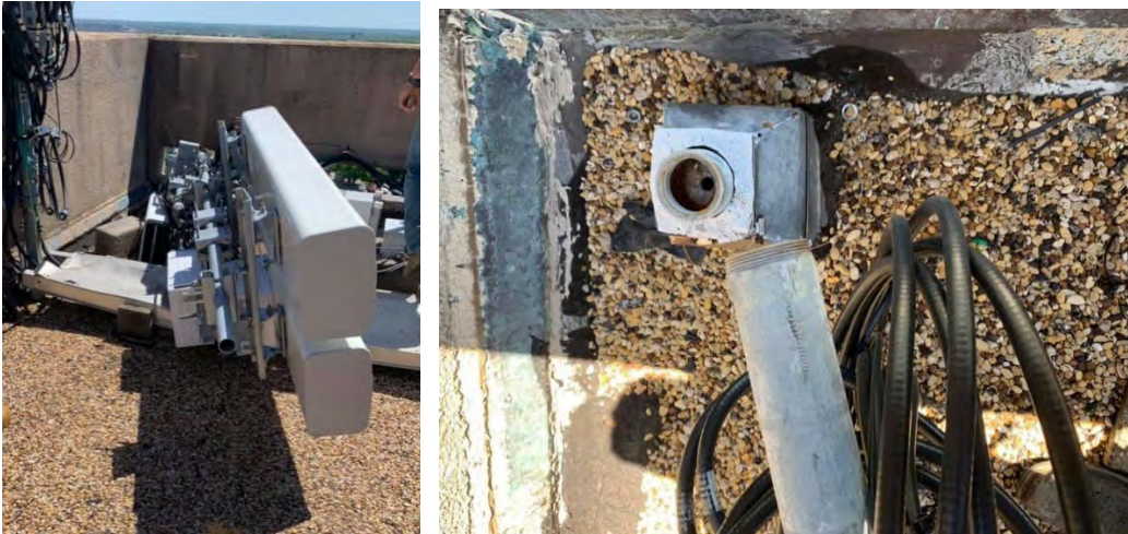
Figure B.4: Parapet Panel antenna mount failure due to improper anchorage
