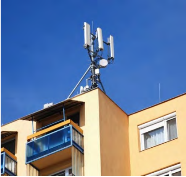
Figure A.d.3: Small Monopole Tower installed on a building roof
