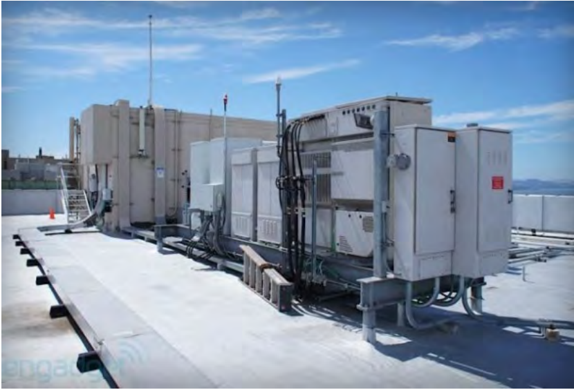
Figure A.c.1: Custom equipment platform
