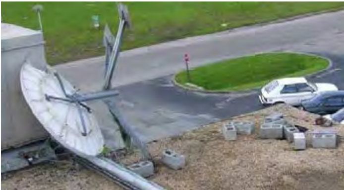
Figure B.2: Rooftop satellite Dish overturned as a result of not having enough CMU blocks and blocks not properly placed. (Ref: FEMA 543 )
