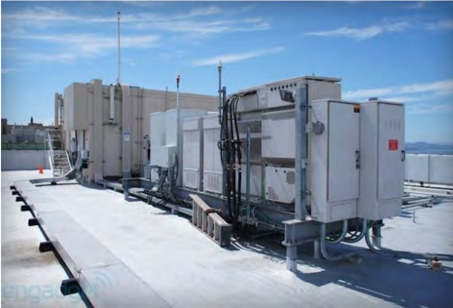
Figure A.c.1: Custom equipment platform
