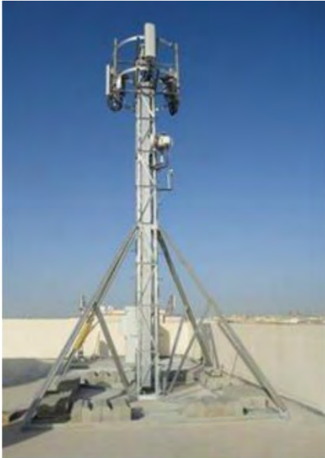
Figure A.d.1: Small Lattice Tower ballasted on corner of a building roof
