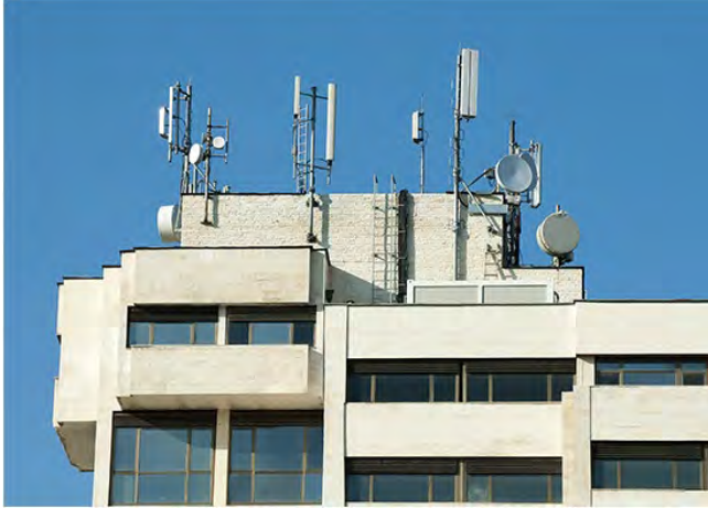
Figure A.a.3: Different types of wall mounts installed on the penthouse wall of a building
