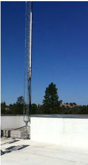
Figure A.d.2: Small Lattice Tower ballasted on corner of a building roof
