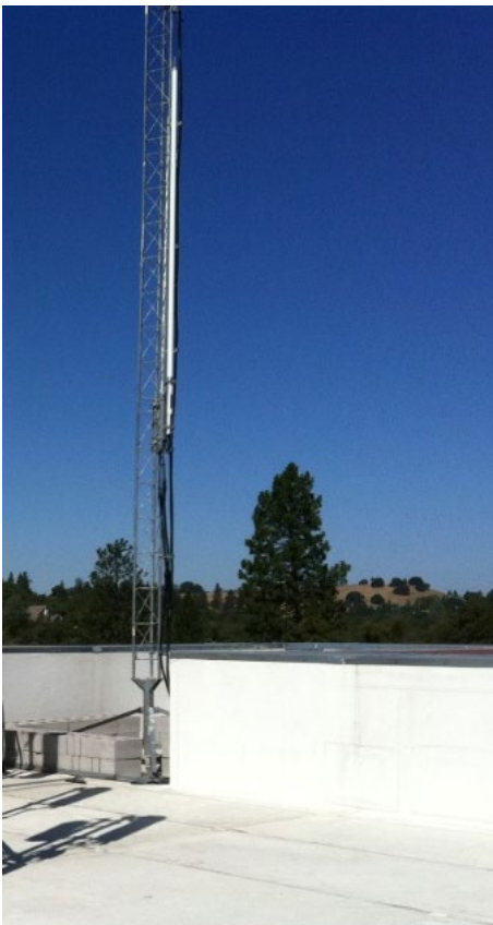
Figure A.d.2: Small Lattice Tower ballasted on corner of a building roof
