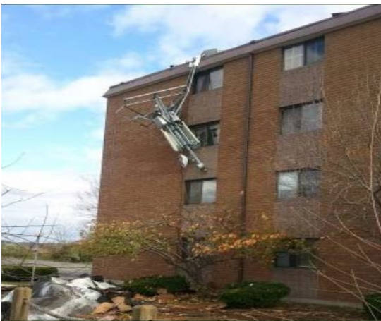
Figure B.3: Rooftop tripod mount fell off the roof as a result of not having enough CMU blocks or proper anchorage
