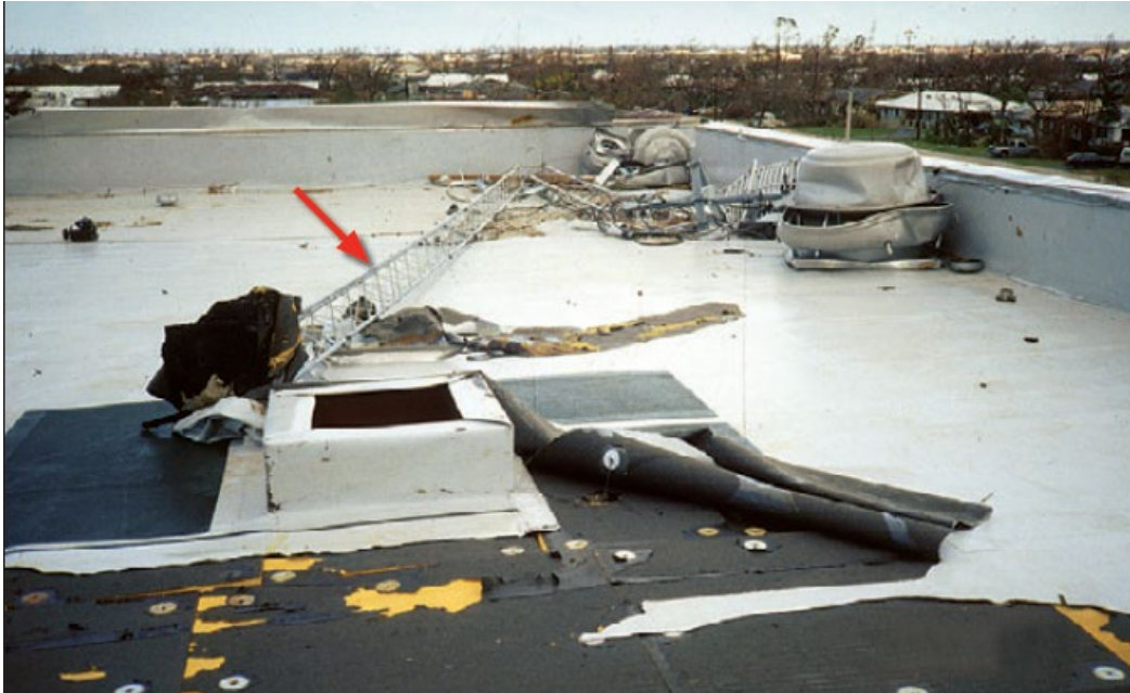
Figure B.5: Collapse of roof mounted antenna tower including progressive peeling of the roof membrane (Reference: FEMA 543 Risk Management Series: Design Guide for Improving Critical Facility Safety from Flooding and High Winds (January 2007))
