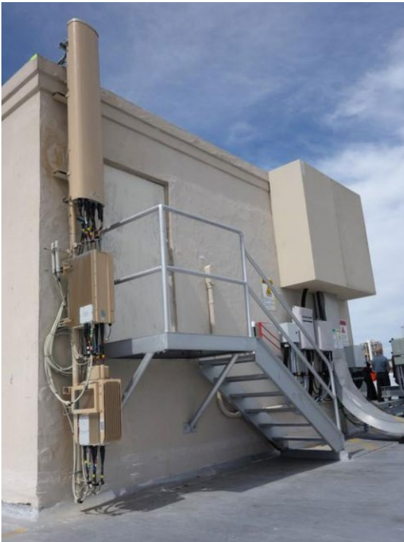
Figure A.a.2: Wall mount installed on the penthouse wall of a building
