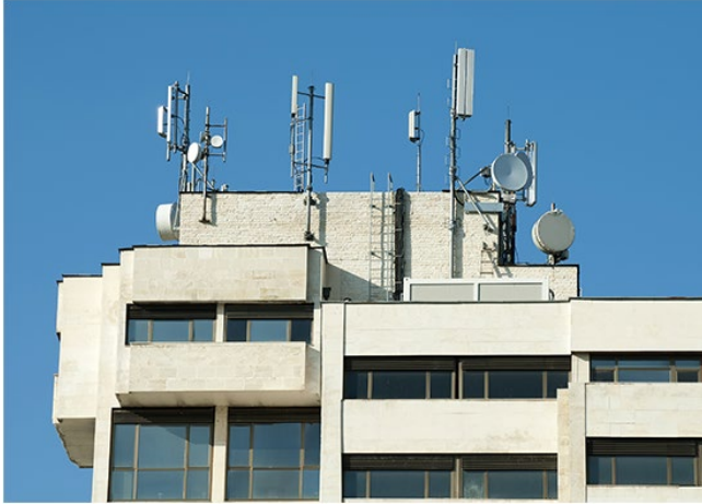
Figure A.a.3: Different types of wall mounts installed on the penthouse wall of a building
