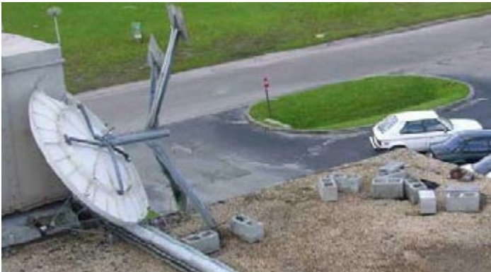
Figure B.2: Rooftop satellite Dish overturned as a result of not having enough CMU blocks and blocks not properly placed. (Reference: FEMA 543 Risk Management Series: Design Guide for Improving Critical Facility Safety from Flooding and High Winds (January 2007))
