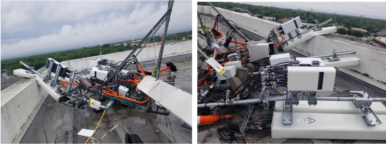
Figure B.1: Rooftop sled-mount frame overturned as a result of not having enough CMU blocks
