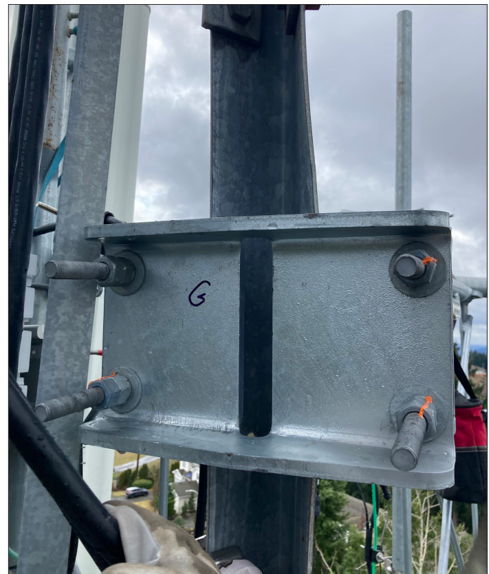
Figure 2: Installation Fault due to over-tightening of clamp resulting in leg warping
