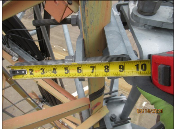
Figure 1: Example where calculated torsional failure was identified
