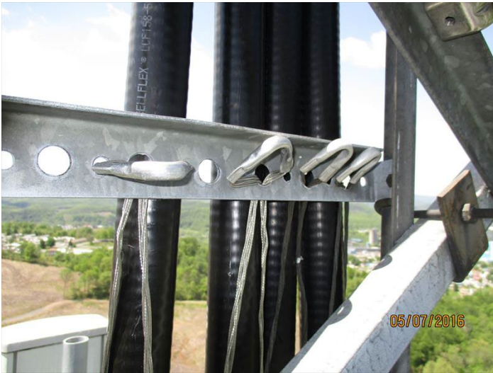
Improper use of grip – Grip was not used to hoist the line and too many lines at one location.
