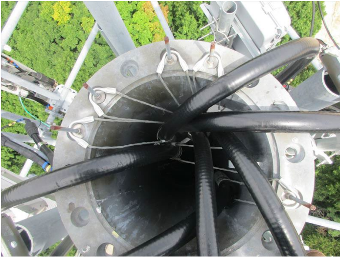
Example of a poorly selected anchor point
